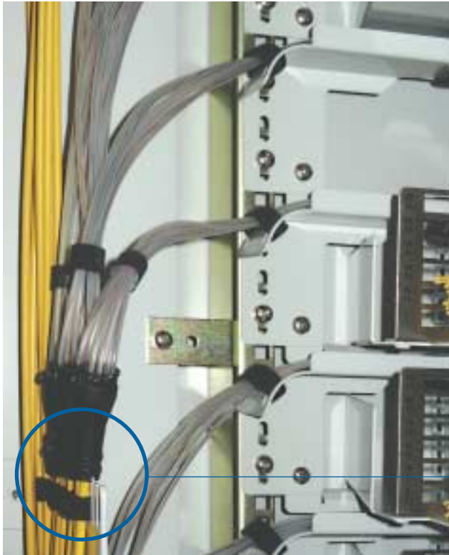
The protected fibers go to the swing out module and safely enter the splice cassette.
