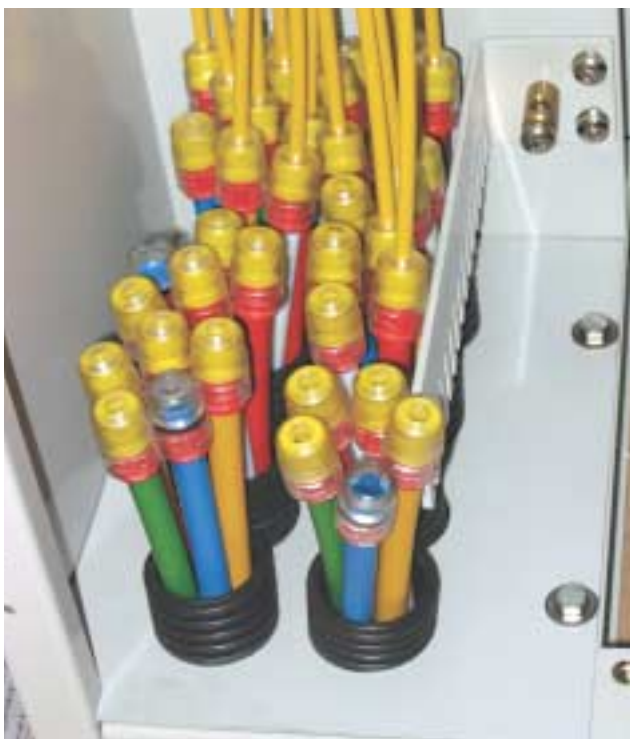
Tubes or cabling entering at the left bottom side.
